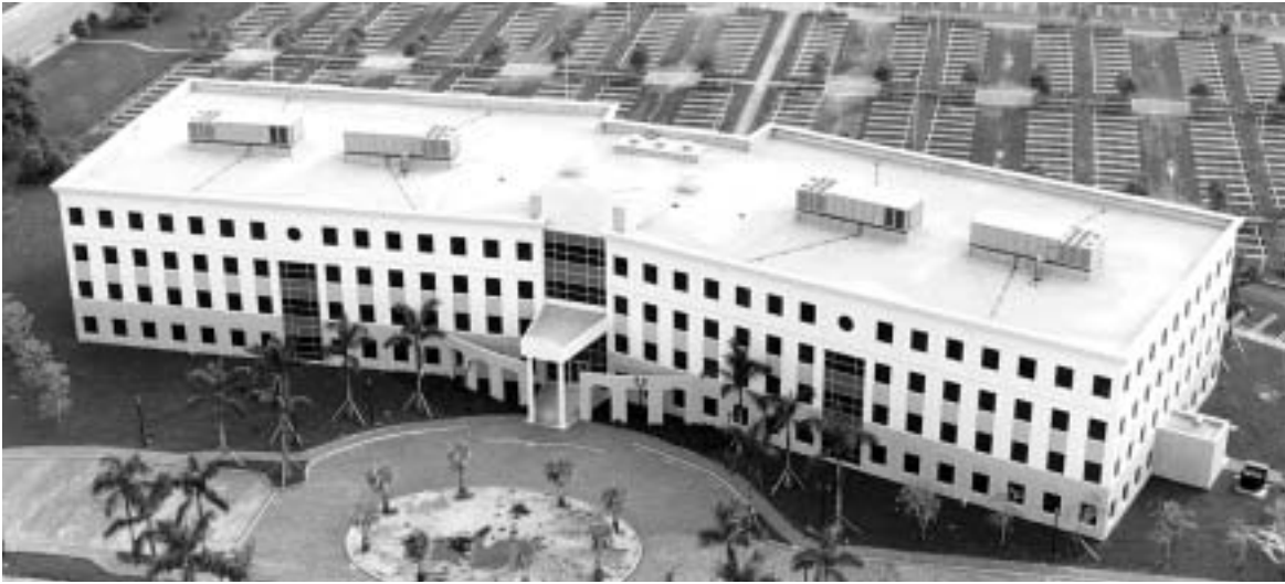
AA Advance Air installed four 130-ton rooftop units on top of the new Doral Costa Office Building in Miami.
